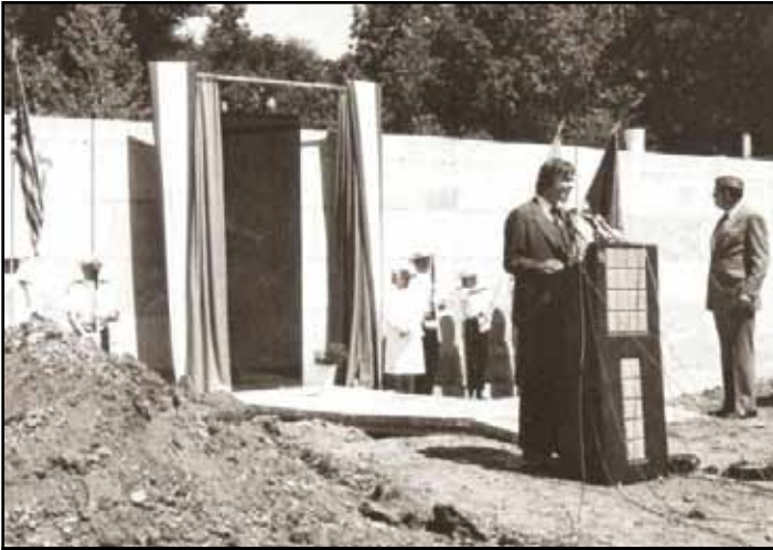
Emogene Cupp, PNP, installing the first panel of The Wall. Jan Scruggs, Founder of the Vietnam Veterans Memorial Fund is in the foreground. July 22, 1982.
